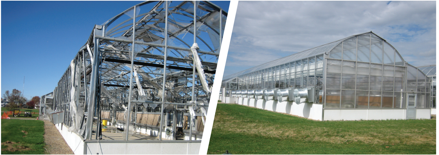
Gourley Greenhouse, OARDC Wooster, Ohio after tornado damage, and the repaired structure with new curved glass roof.
